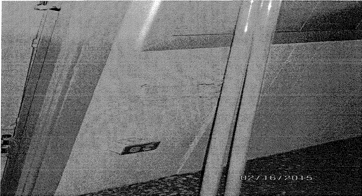
Figure No. 11 Date Taken: 2-16-15 Facility: Manuel F.L. Guerrero Administration Bldg. Description: Fluorescent lamps located in room #260 former DOE offices 2 nd floor
