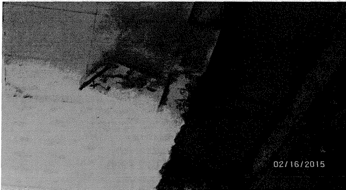
Figure No. 14 Date Taken: 2-16-15 Facility: Manuel F.L. Guerrero Administration Bldg. Description: Potential mold in former DOA offices 2 nd floor
