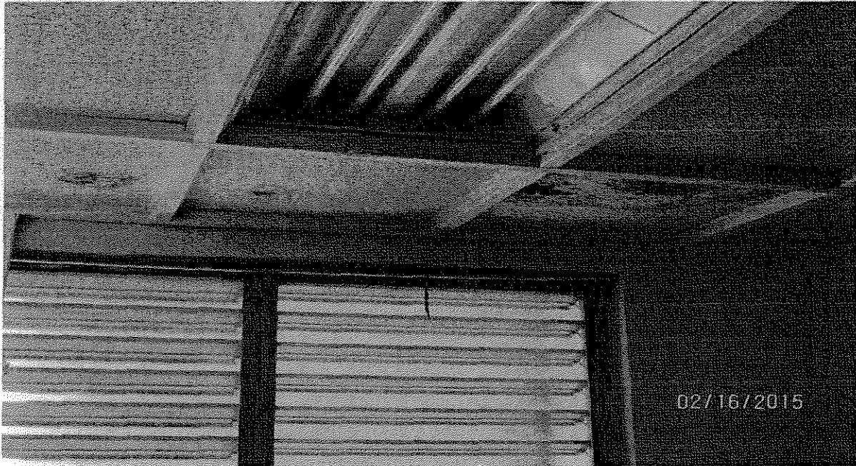
Figure No. 13 Date Taken: 2-16-15 Facility: Manuel F.L. Guerrero Administration Bldg. Description: Potential mold in former DOA offices 2 nd floor
