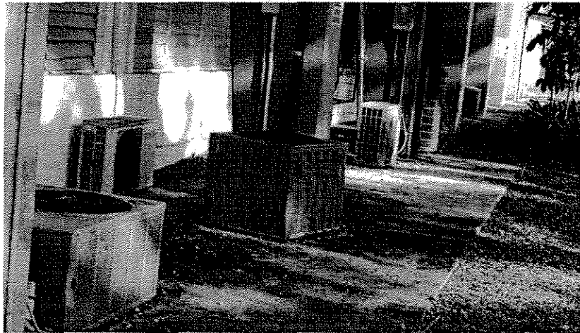
DOA First Floor Corroded and not functioning AC Ventilation
